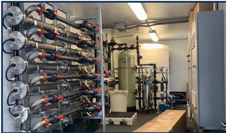
Figure 2: Interior of completed system
