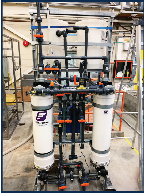
Figure 3: Ultrafiltration skid at UBC
