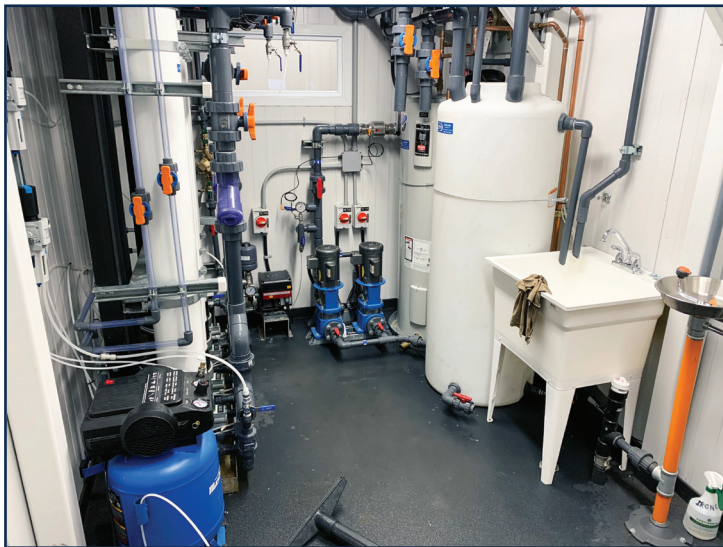
Figure 2: Interior of completed system
